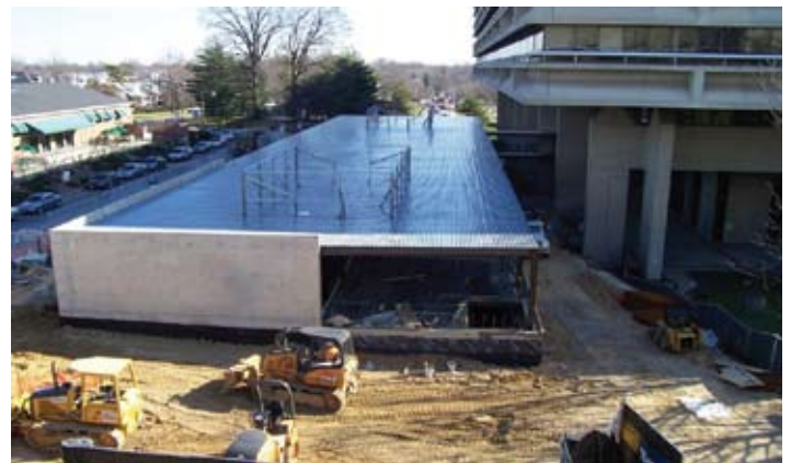
▲ One of the new buildings constructed on the campus was a new Amputee Center. The modern structure was designed to provide a focused area for soldiers to regain skills and return to active lives.
