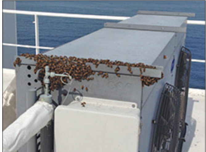
Figure 5. Bee swarm on air conditioning unit aboard USNS Comfort (TAH-20) in port in Acajutla, El Salvador. Photo courtesy of LCDR J. Dunford.
